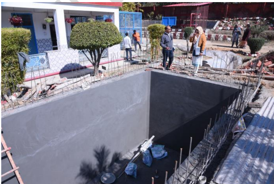
Plate 8: Rain water harvesting pits in the premises
