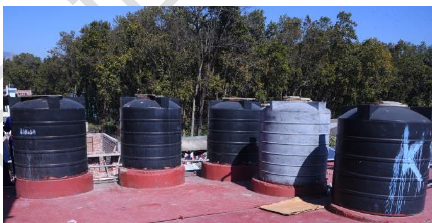
Plate 6: Overhead water tank in the premises
