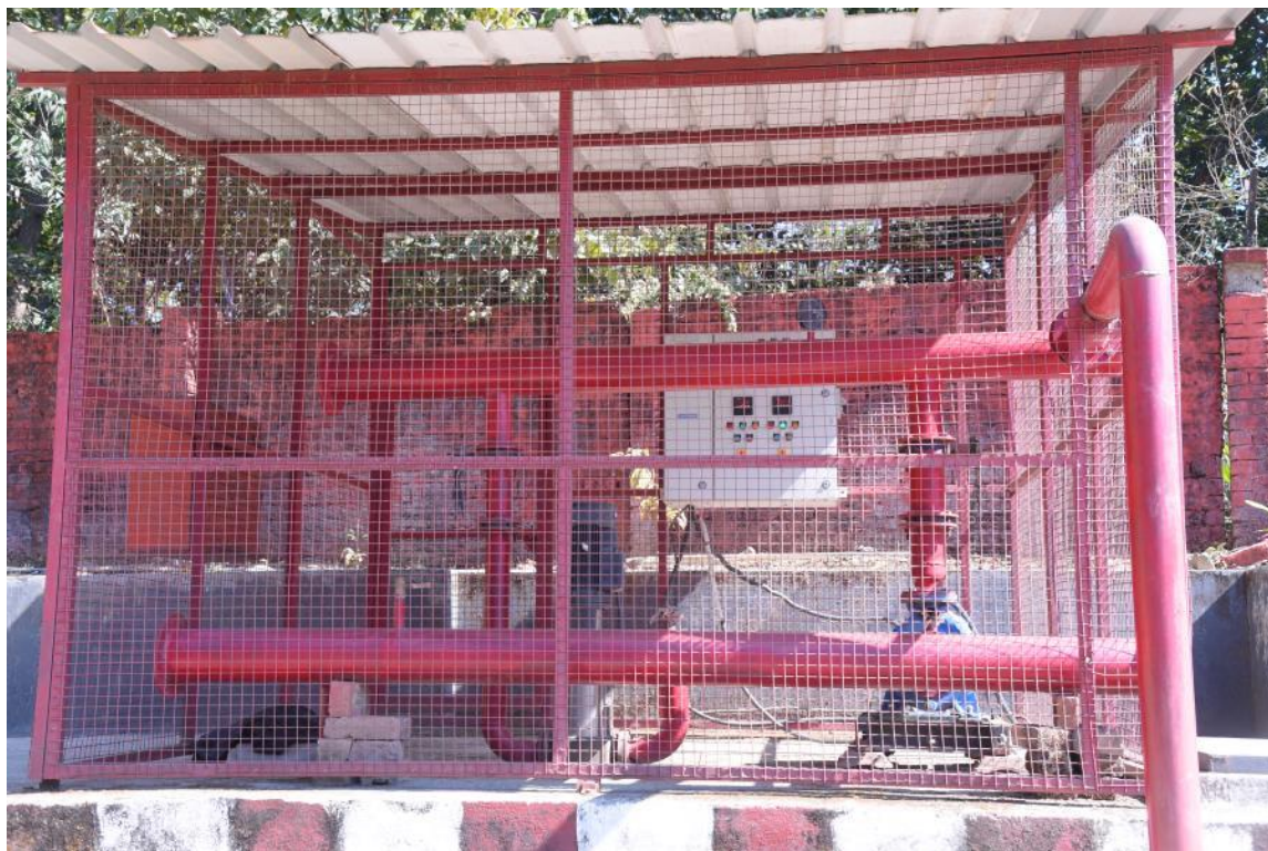
Plate 10: Fire zone with all measures in backyard area of premises
