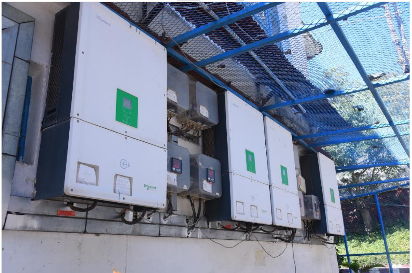
Plate 4: Net metering system in the premises
